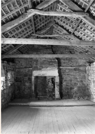
North Gatehouse interior roof modern but some old timbers have been re-used
