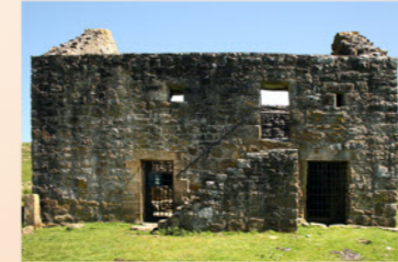
Front (south-west) wall facing across the Tasset Valley; two small windows very restricted view; later ground floor doors and stone stairway
