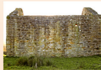
Back (north-east) wall with small window on upper floor; ground floor window, formerly a ventilation slit, now blocked
