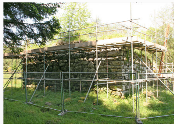
Conservation work at Boghead Bastle English Heritage recently funded work on Boghead and Shilla Hill bastles; vegetation has been cleared, masonry consolidated
